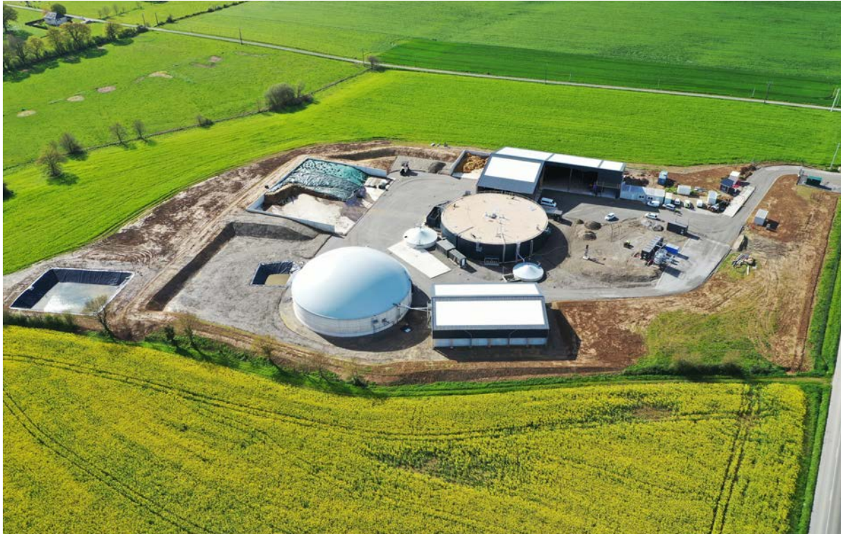
Picture: BIOGEST 135 Nm 3 /h (41,857 MMBTU/year) PowerRing biomethane plant in Congrier, FR (Photo by M. LEBIHAN BSVL)
